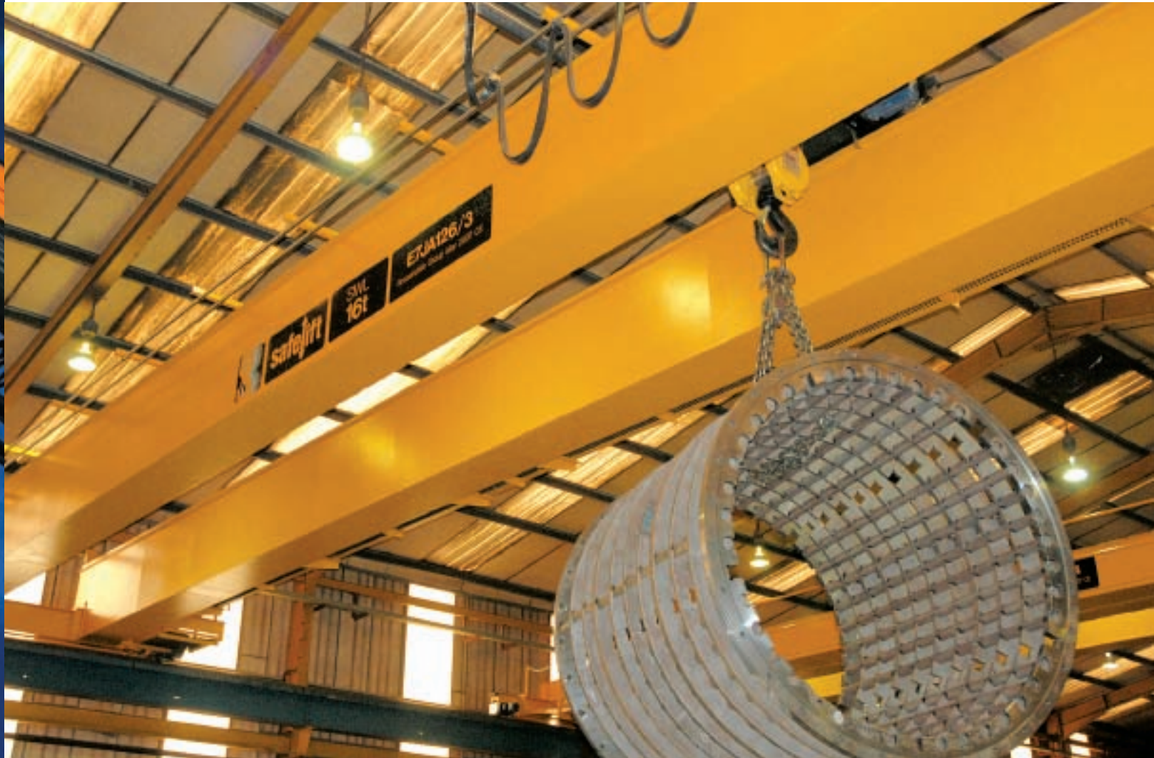
Above Safelift Overhead Crane
